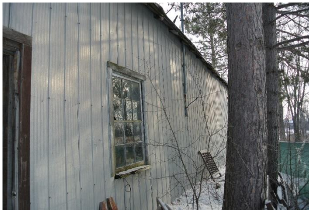
Image 12: View of the six-over-six window on the south elevation of the one-and-a-half storey accessory building.
