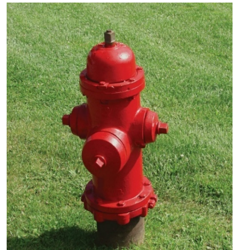
Figure 28: Picture of Private Hydrant
